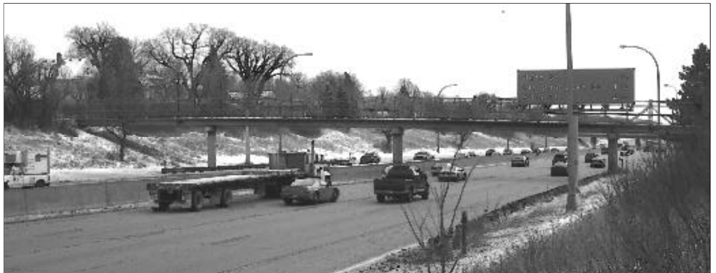
The King Bridge Partnership is working to replace the current substandard pedestrian bridge at 40th Street
